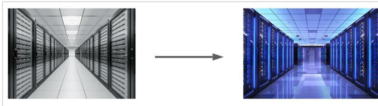
Figure 1: Relocation — from One Data Center to Another
